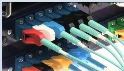
Patchcordy LC Secure w panelu
